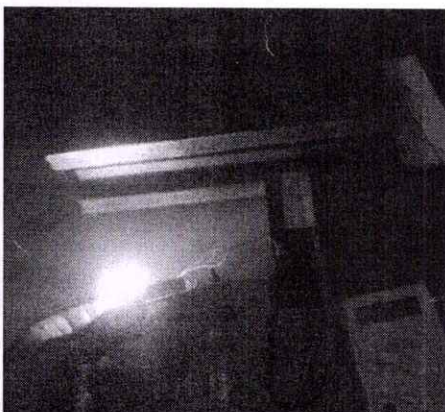
Figure 6: Connected a DC LED load.
